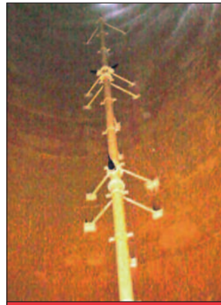
TMS Vertical Riser with Tideflex® Diffuser Nozzles Installed in Mono Mills
